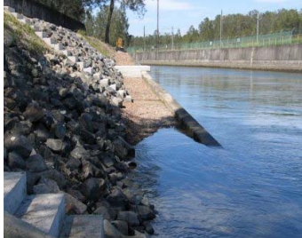
Turtle embayment area at Eraring Power Station inlet canal
